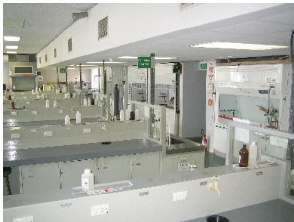
New fume hoods in Chemistry Laboratory
