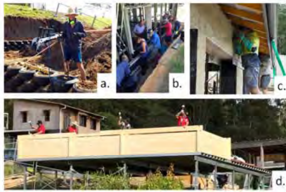
Figure 3 - Building technologies of homes 1 to 4. a. Compacting earth in tyres -earthship home 1 (Source: S. Bozkewycz); b. Home 2 volunteer hempcrete wall workshop (Source: G. Cameron); c. Home 3 hemp walls by builders (Source: M. Ong); d. Home 4 builders hammering together the solid timber wall (Source: P. Atkins)
