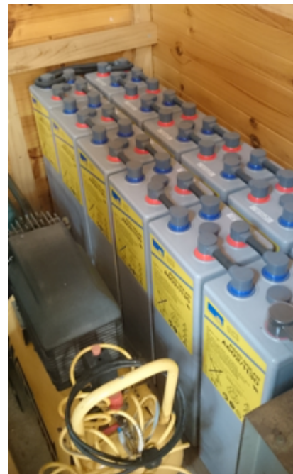
Plate One: Battery array in Tasmanian off-grid household
