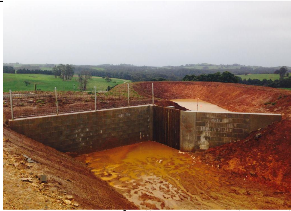
Effluent system up grades - 120m 3 trafficable solids trap (concrete floor) with weeping wall draining into an expanded 2ML storage pond. Liquid effluent will be applied to paddocks via a 3" hard hose irrigator
