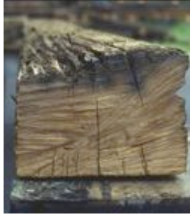
A weathered bridge deck element
